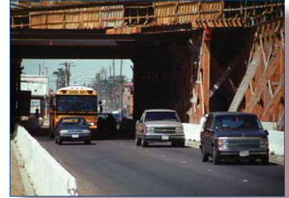
Image courtesy of the APWA Jim Martin Public Works Photo Library at www.apwa.net .
