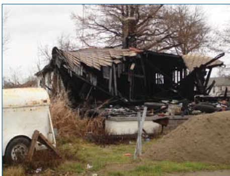
Image of post-Hurricane Katrina damage taken during a visit by the APWA Executive Committee in 2007.
